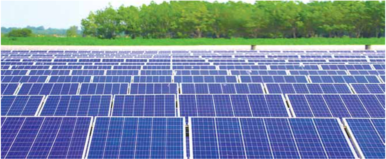
Dau Tieng 3 Solar Power Plant
