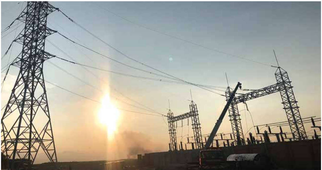
Connecting the 110kV the line to Son My 3.1 Solar Power Plant Substation
