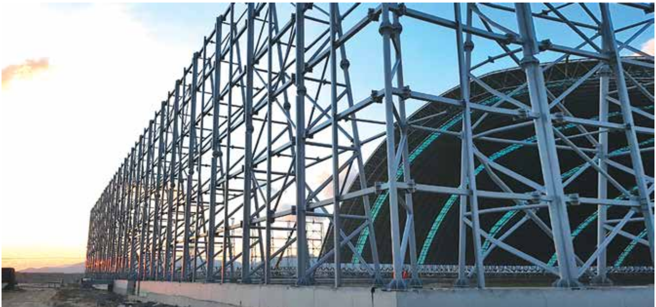
Vinh Tan 4 Extension Coal Yard
