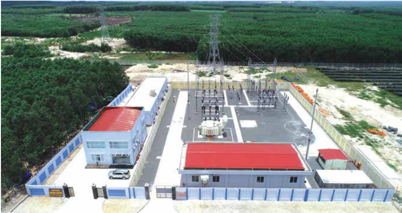
Son My 3.1 Solar Power Plant Substation
